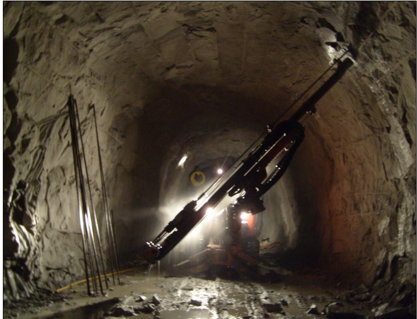
Lake Dorothy hydropower project, Juneau , Alaska
